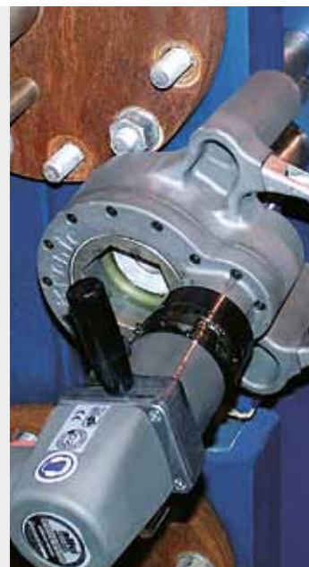
Image above: PWT of Alfa Laval Images on the right: alkitronic ® CLS-SG and RCL in operation on plate heat exchangers.
